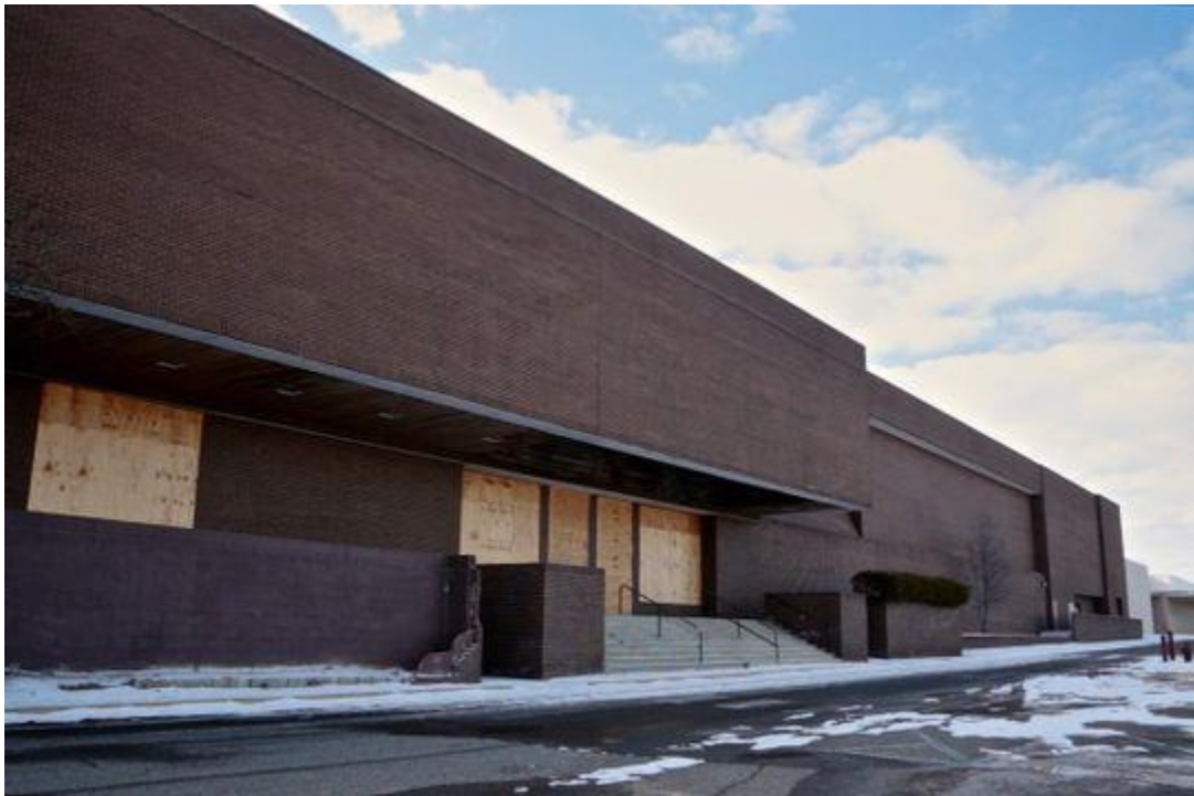
Northland Center mall is seen on Wednesday, February 17, 2016, in Southfield, MI. (Photo: Salwan Georges, Detroit Free Press)
