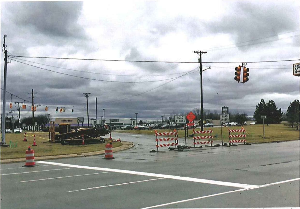
The 3.9-mile redo of M-59/Hall Road between M-53 and Romeo Plank Road in central Macomb County will close lanes up and down the length of construction for the next two summers.
